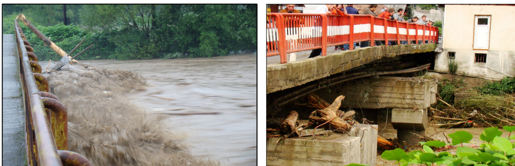
Figure 7. Bridges affected by flood in Vişeu de Sus town, July 2008.
